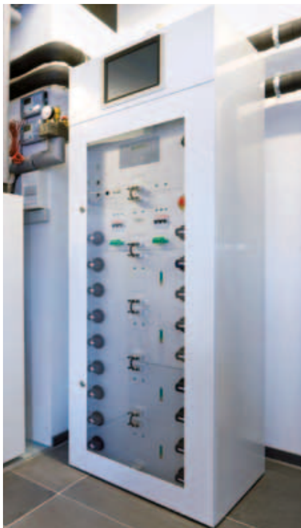
Newer battery storage, 13.2 kWh
