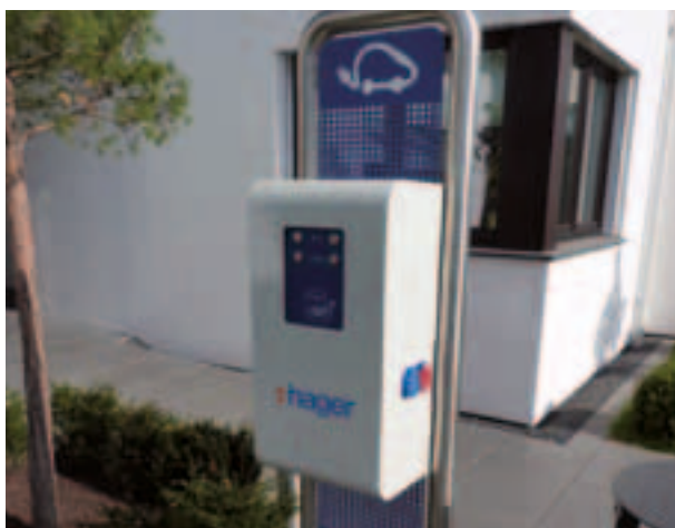
Electric vehicle charging point
