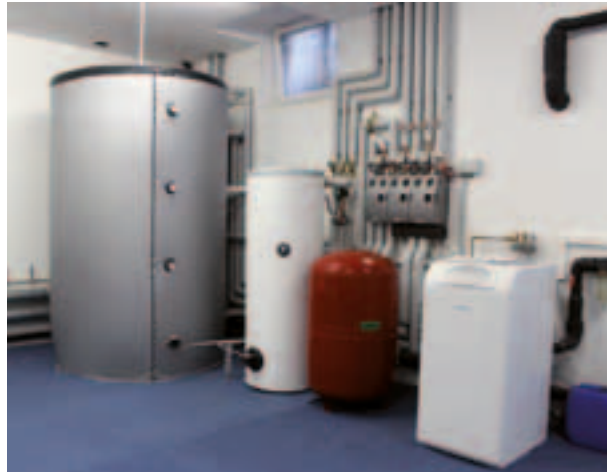
Heat pump system with buffer storage tank (5 000 l)
