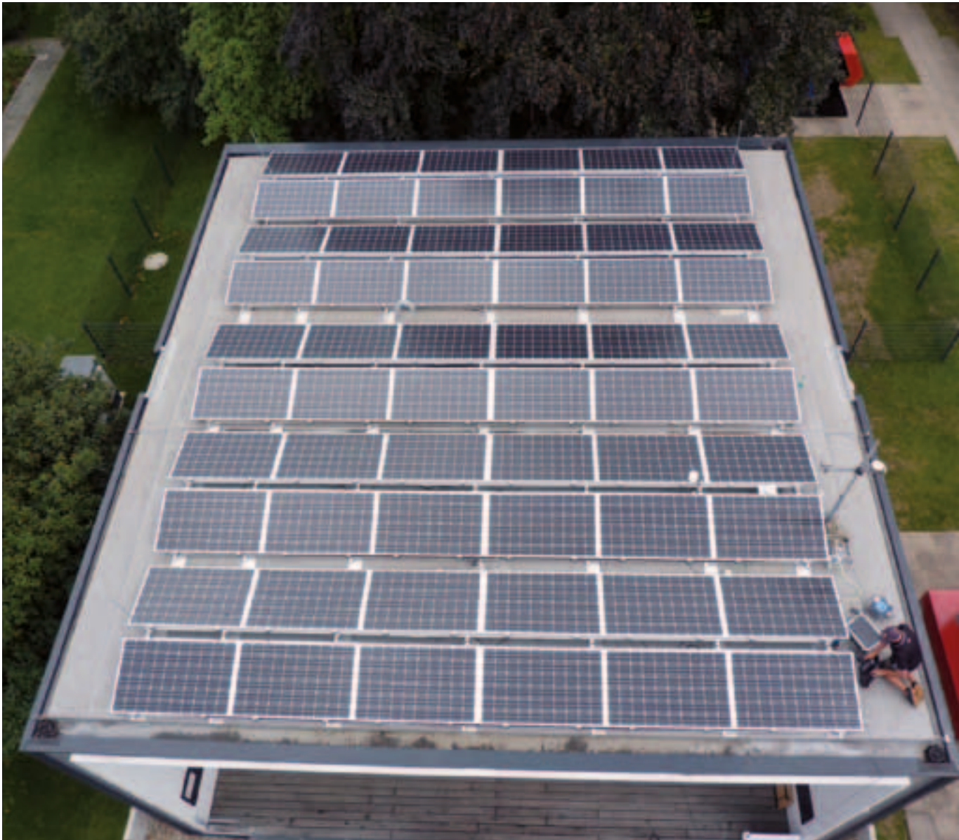
Roof with monocrystalline photovoltaic modules
