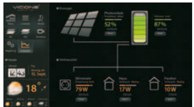
A display screen in the building automation system
