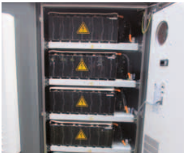
Battery bank consisting of used car batteries, 40 kWh
